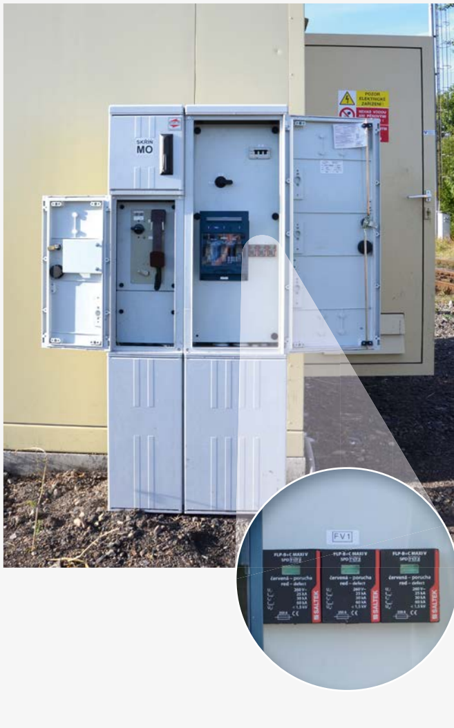
Fig. 2 View to power distribution box of signalling system with installed SPD, type 1+2 FLP-B+C MAXI V/3
